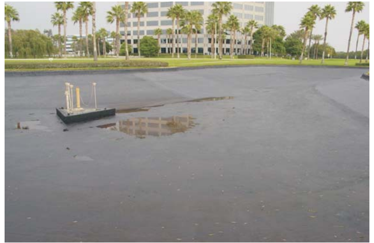
The WeatherWeld Seamless Composite system was then applied in two total passes of 30 gallons of emulsion and 16 pounds of multi-filament fiberglass roving.
