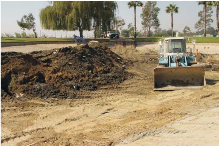
A front end bob-cat loader removed the final layers of debris and the ground was then compacted.
